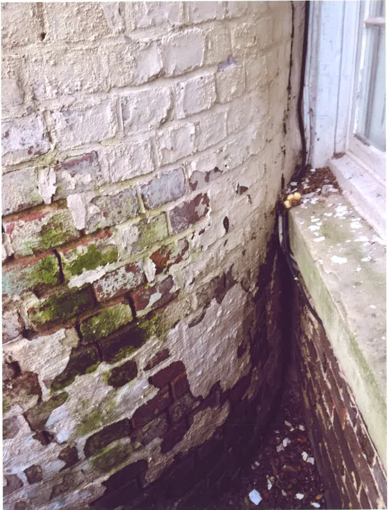
Photo 6 Current detail of exterior wall of curve and intersection with original rear wall of dwelling
