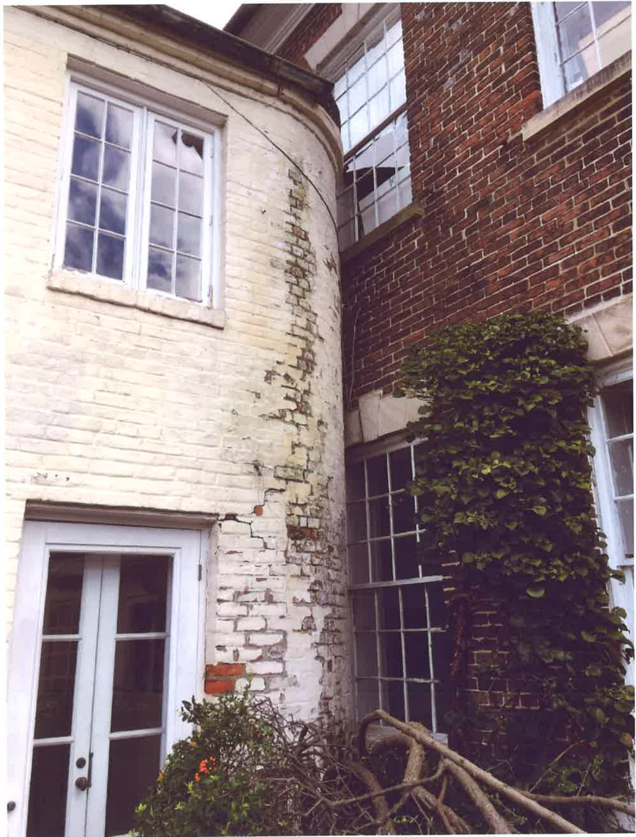
Photo 3 Current detail of exterior wall of curve and intersection with original rear wall of dwelling
