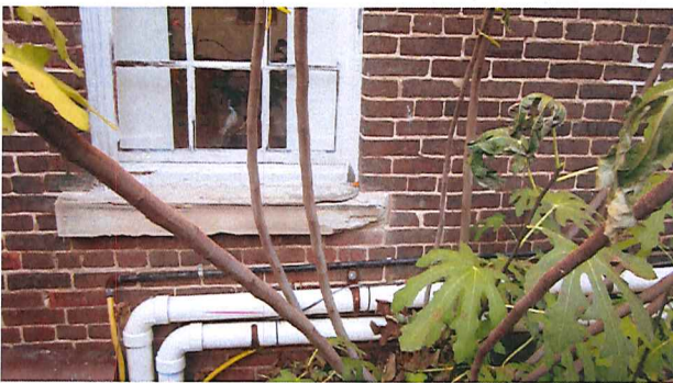
2 DAMAGED STONE SILL - REPAIR OR REPLACE NOT TO SCALE
